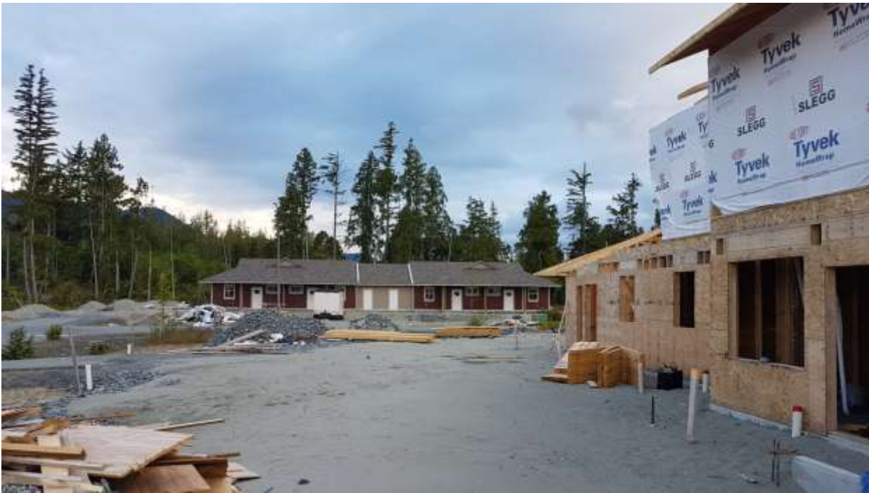
Picture: Six plex housing complex looking north toward the four unit Teacherage
